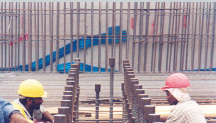
Bartec/Fortec couplers in columns
